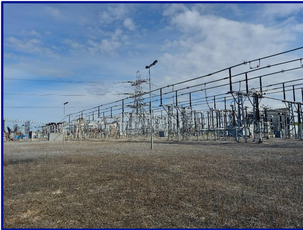
Figure 2: Existing Substation - Monk Fyston (Source: MM Site Visit)
